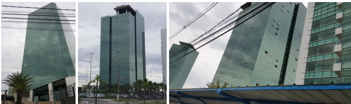
Figure 11. Full-scale damage to cladding elements: some windows that were not locked were destroyed
