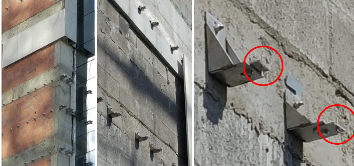
Figure 14. Full-scale damage caused by downburst and granite plate supporting system
