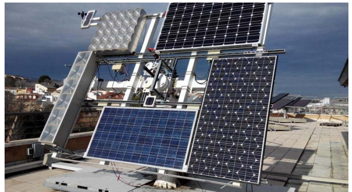
Fig 3. Solar tracker installed at the University of Jaen for the characterization of different PV modules in RSC.
